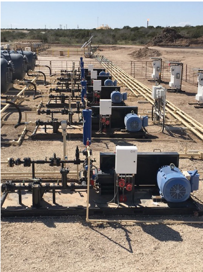
Sample well site showing JJ Tech's seal-less pumps, no fluids, no leaks.
