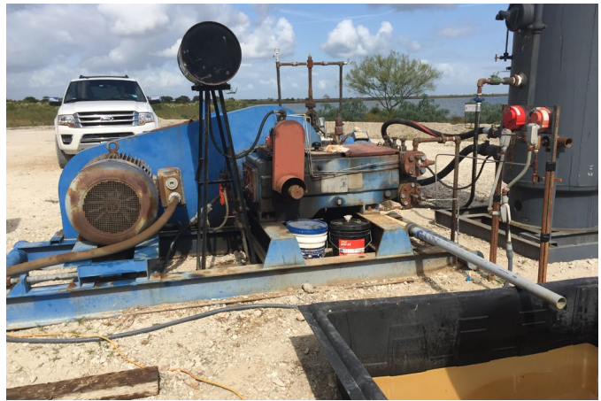
BEFORE | Oil and water leaking out of pump into tub.
