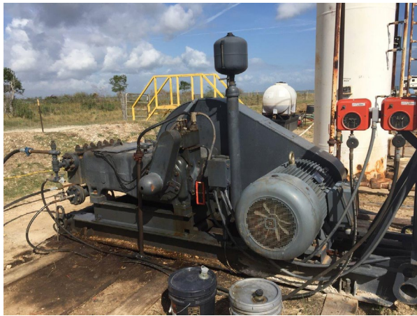
BEFORE | Oil leaking on the ground
