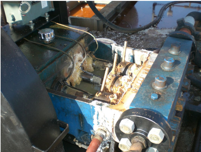
Typical triplex pump leaking saltwater
